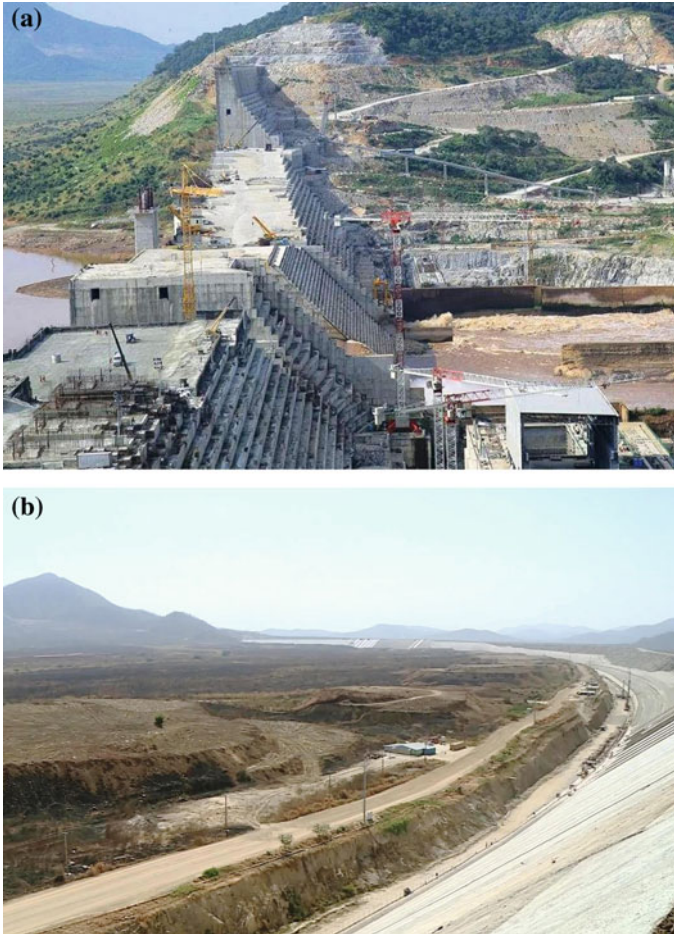
Fig. 6.4 a GERD RCC gravity dam showing the main dam and the left side power house under construction; b concrete faced rockfill saddle dam (2018)
